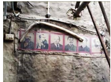
Gutted house of Comrade Sudhanshu Jana in Moipith
